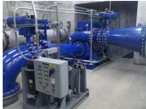
The Canyon Hydro Francis-type turbine fits into the existing water treatment facility for the City of Logan, Utah.
