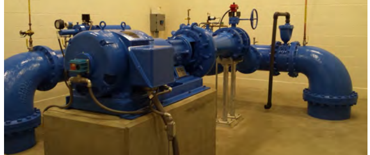
A turbine and generator (on pedestal) similar to what's to be installed at Covington.
