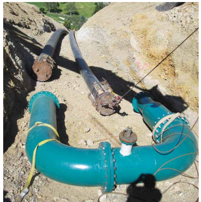
The U-shaped return is installed at the top of the surge pipe
