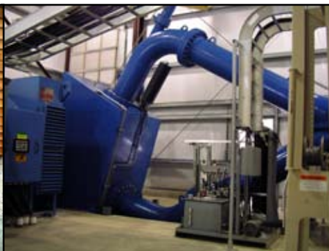
Canyon Hydro turbine inside the powerhouse
